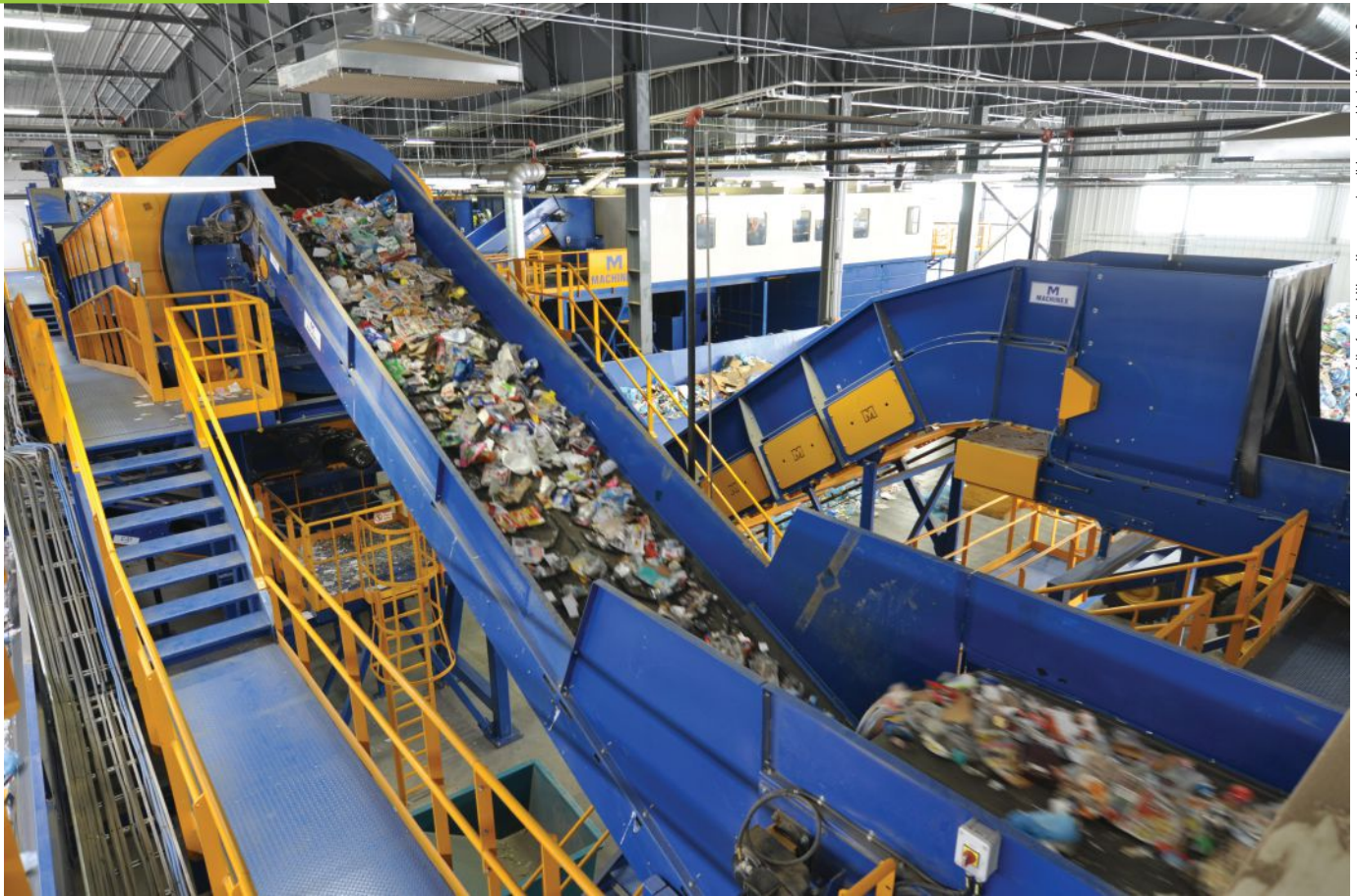
Central Newfoundland Waste Management, in collaboration with the Machinex Group
